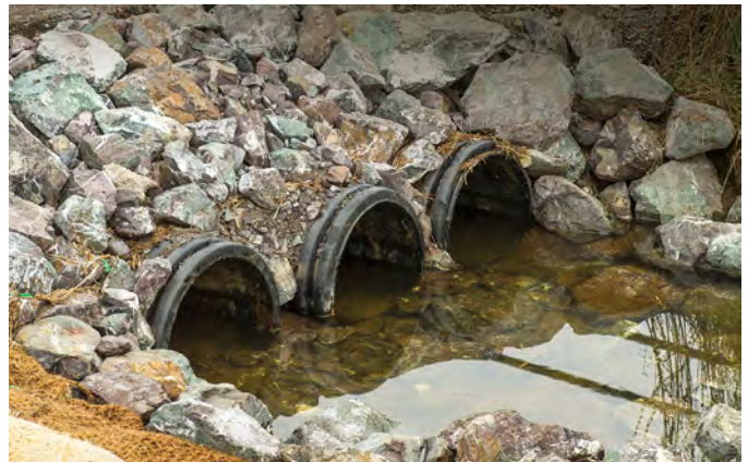
These culverts are part of the newly constructed Willits Bypass on U.S. Highway 101.
